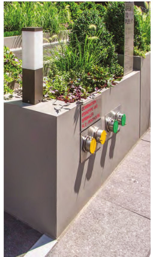
Service areas should be designed to be compatible with the architecture of the rest of the development.
